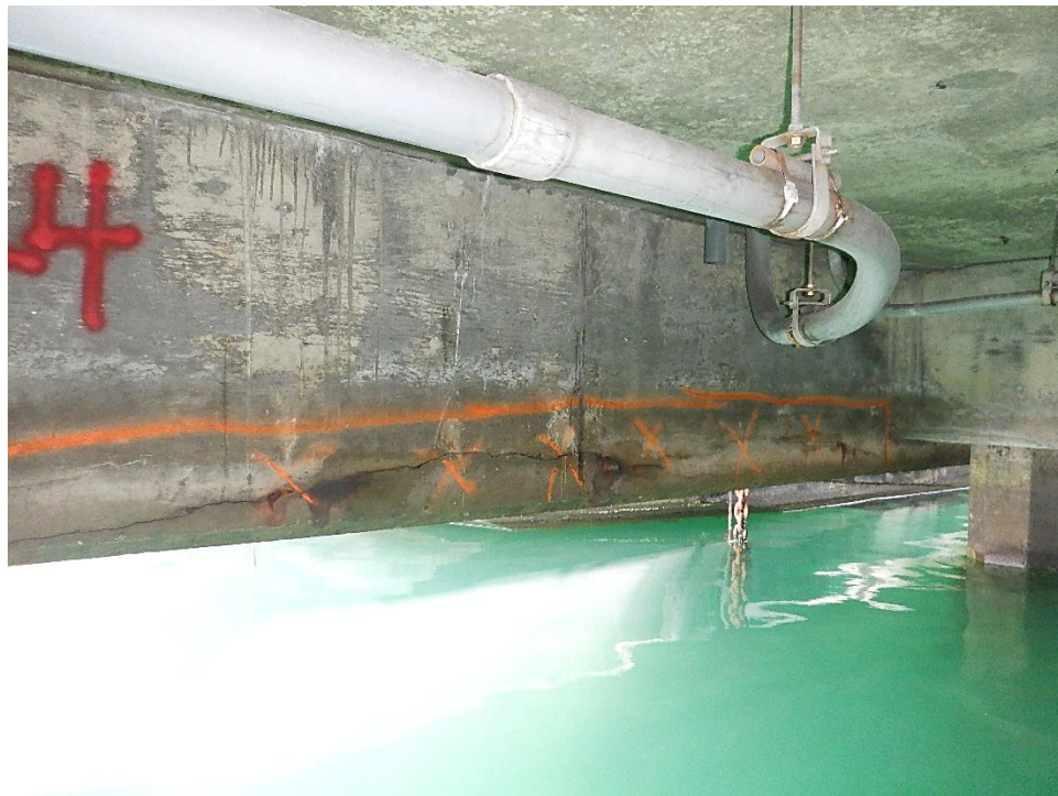
Photo 6: Typical Fascia Beam Spall at Pier 17
