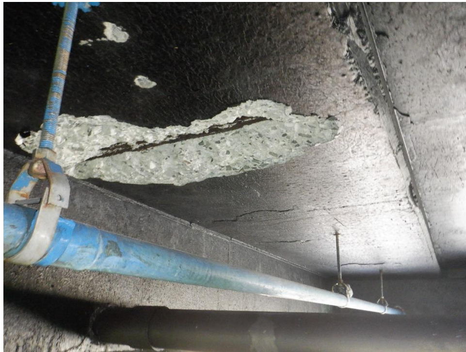
Photo 2: Typical Precast Plank Soffit Spall at Pier 16
