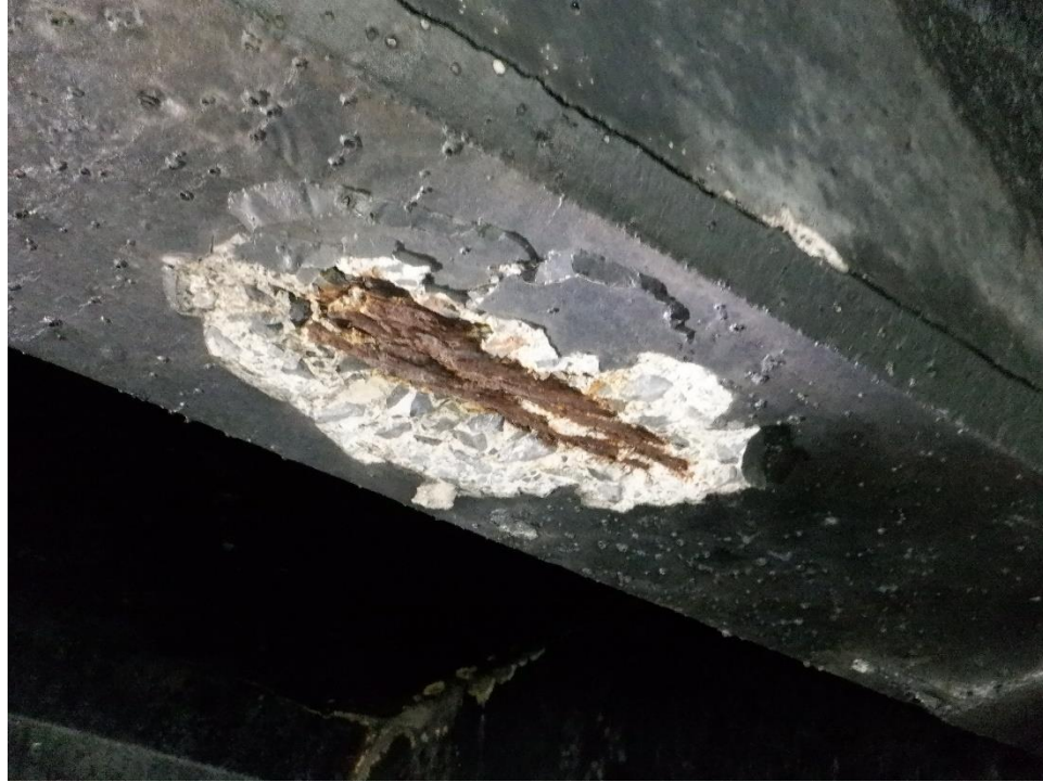
Photo 3: Typical Precast Tee Beam Spall at Pier 16
