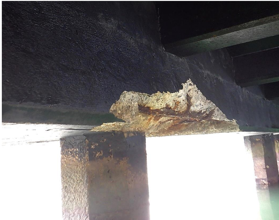
Photo 4: Typical Fascia Beam Spall at Pier 16
