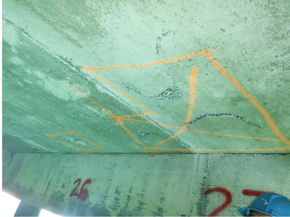
Photo 5: Typical Precast Plank Soffit Spalls at Pier 17
